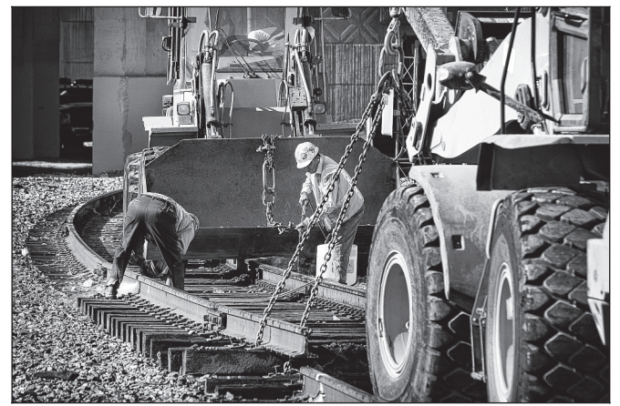
Railroad workers remove old tracks near the Colton Crossing. The fly-over, featuring two tracks, runs parallel to Interstate 10 from Rancho Avenue on the west to Mt. Vernon Avenue on the east.
